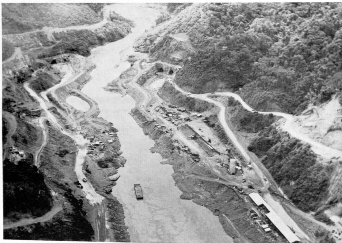
Raudales Dam, a panoramic view showing four of the five tunnels constructed. Flood control will be made by a controlled crest spillway and floodgates.
