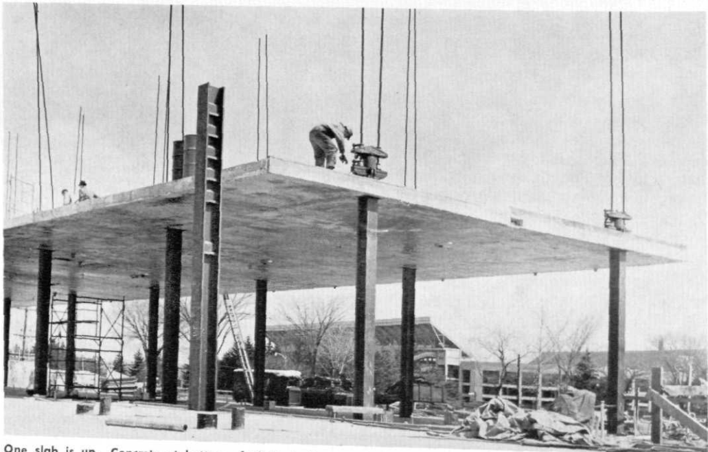
One slab is up. Concrete at bottom of photo is the next floor ready to go up. Note the circular cans set in the slab to create openings for pipes. (MSU Information photo)
