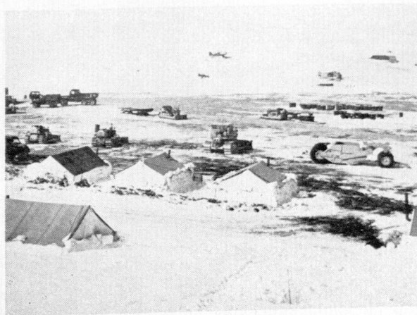
Top of the world — Bush planes land on the frozen snow to supply lonely construction camps like this one. Some of these bases are only ten minutes by air from Russia.
