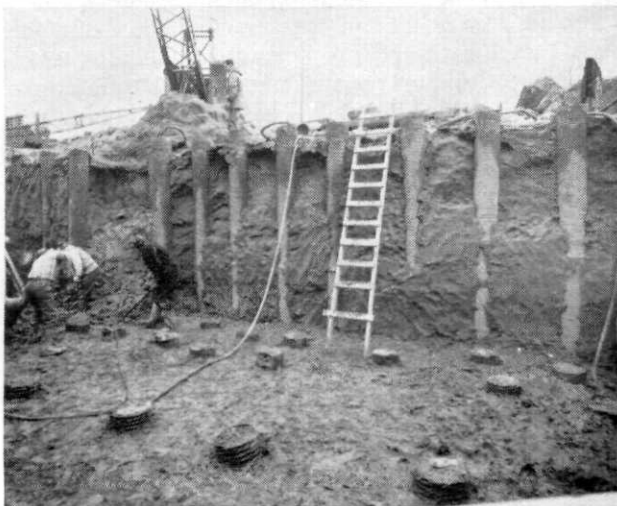
HERE'S WHAT SOUPY SILT looks like after being treated with electro-osmosis. The intake tunnel is being excavated with clamshell and clay spades, walls standing straight up without shoring or bracing.
