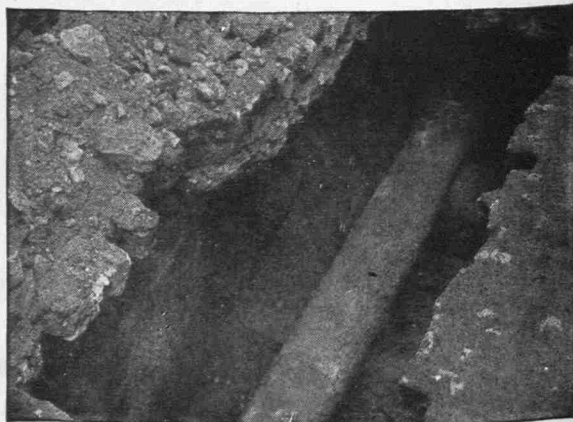
Section of 114-year-old cast iron gas main still in service in Baltimore, Md.
