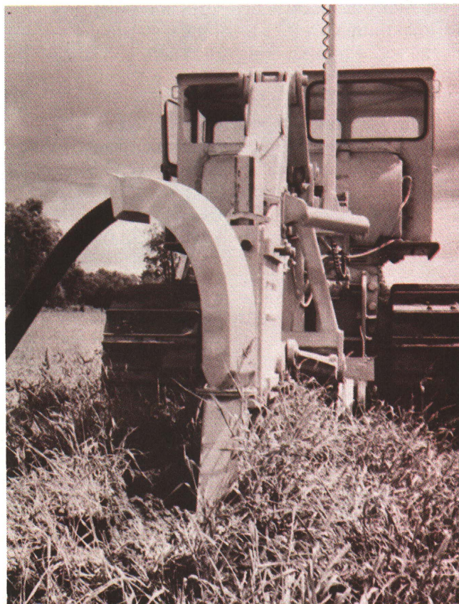
Figure 9. The mole plow is now used extensively to "plow in" to the soil corrugated plastic tubing. There are many advantages to this method, and some concern because the trench is not observed; hence presence of fine sands and silts cannot be detected until the tiles fill and stop drainage.
