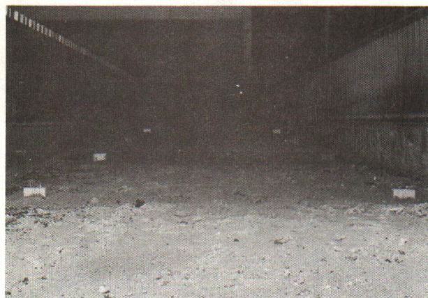
Fig. 5. Stakes in place to give a 2% slope to the floor of the trench.
