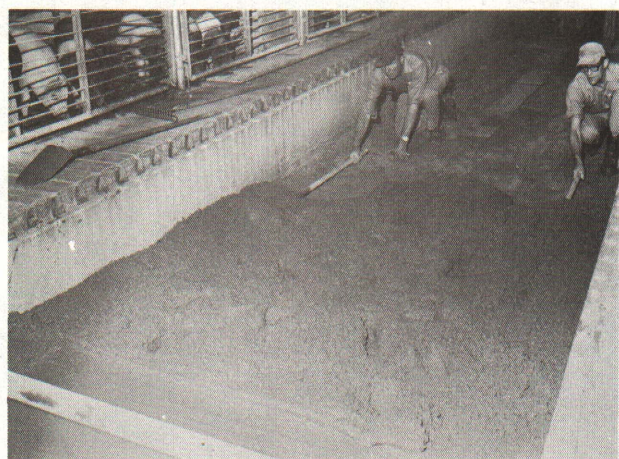
Fig. 7. Moving the pipes as pouring progresses. To maintain an even slope, make sure the pipes are always resting on 3 stakes.
