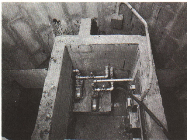
Fig. 8. These two pumps are used to recycle water from a lagoon back into the building for flushing or to pump water for irrigation. The water is taken 4' off the bottom of the lagoon and passed through a screen before reaching the pump.
