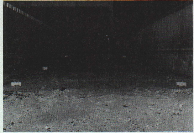
Fig. 5. Stakes in place to give a 2% slope to the floor of the trench.
