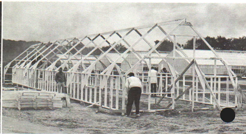
Fig. 3 Framework of the greenhouse prior to pouring concrete around the rigid frames.
