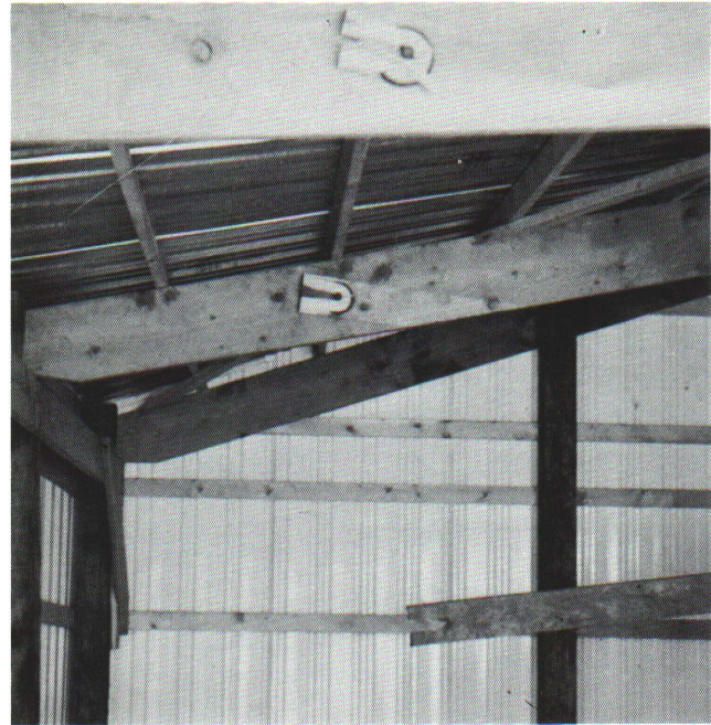
Figure 2 — One-2½ in. split ring was used on this joint where at least two rings should have been used.
