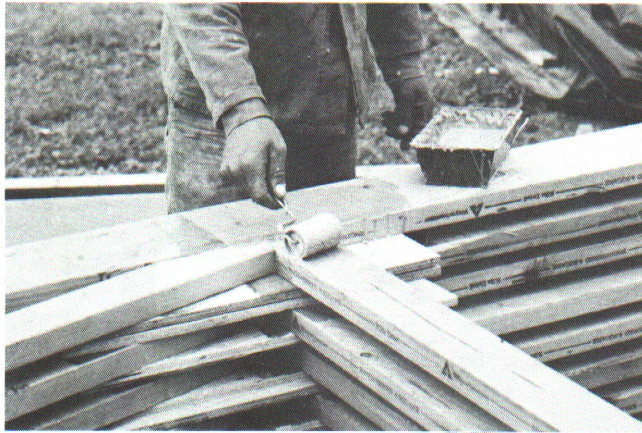
Figure 7 — Applying glue with a paint roller. A paint brush can also be used.
