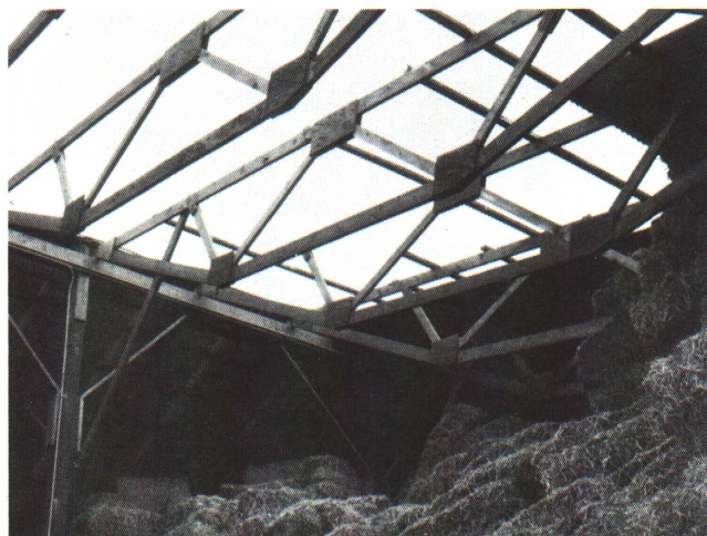
Figure 11 – Poor nailing of roof girts to trusses caused this section of roof to blow off during high wind.
