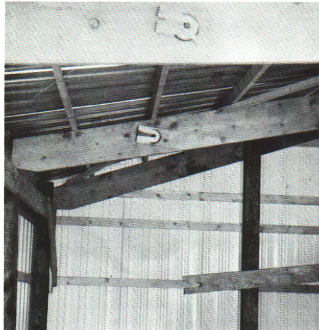
Figure 2 — One-2½ in. split ring was used on this joint where at least two rings should have been used.
