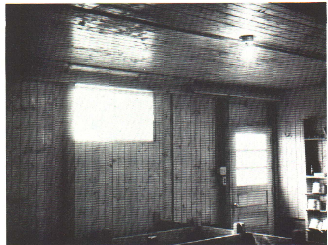
Figure 11 — A 3-inch slot along the ceiling provides space through which dry, cold, fresh air can enter the building. Hinged flaps can be used to deflect the air across the ceiling.
