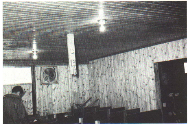
Figure 10 — A ventilation system should include a fan, a timeclock controller and fresh air inlets.
