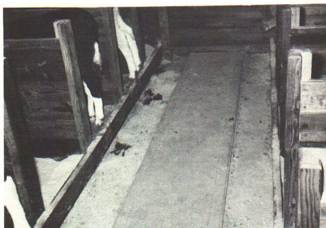
Figure 4—A shallow gutter behind the stalls collects manure and prevents liquids from running into the alley.
