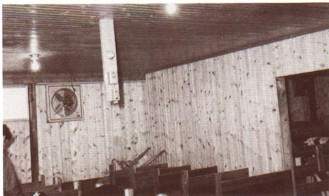
Figure 6 — An exhaust fan mounted in the side wall and controlled by a thermostat removes moist, warm air. Thermostat should not be located over a calf stall or near a heater.
