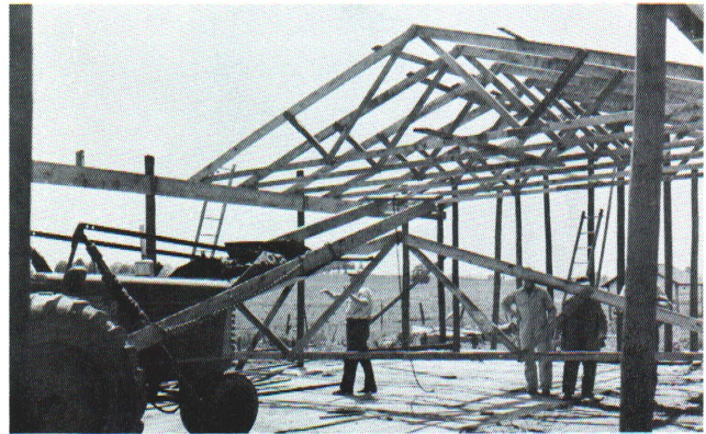
Trusses are raised into position on the building with a farm tractor and loader. An extended frame has been built on the loader to provide for the necessary lifting height.
