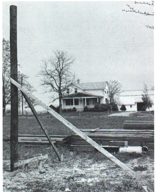
Batter boards are placed at corners. Corner poles set, plumbed and braced in place and chalk lines placed in position.
