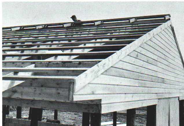
This roof framing and gable end of the pole building has been readied for the application of the sheet metal roofing. A ridge ventilator is being constructed on this building.
