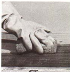
Apply bleach solution with a sponge. Be sure to cover the area completely.
