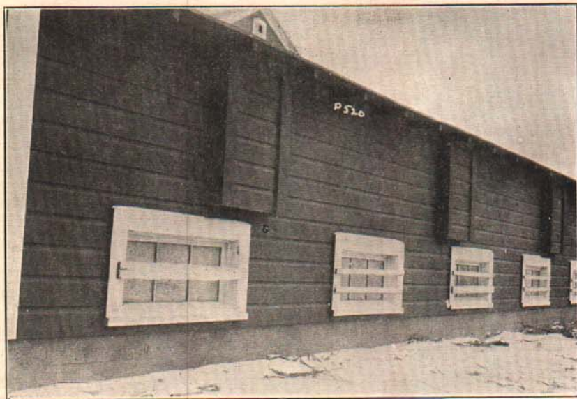
Fig. 9.—Rear Elevation—note the rear windows and the construction of the intake flues.
