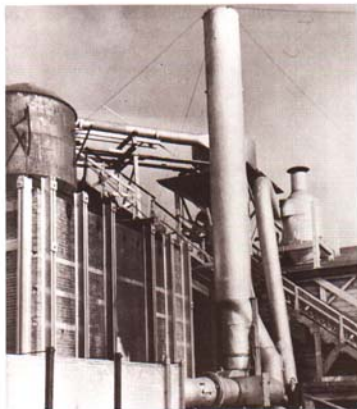
Fig. 30. The second step in converting wet wood waste into fuel briquets involves drying the previously hammermilled refuse in flash driers. The first stage of a two-stage dryer is shown here. See Item 19 in Fig. 27 for the location of this tower. (Photo: Sumner Iron Works, a division of The Black Clawson Company).
