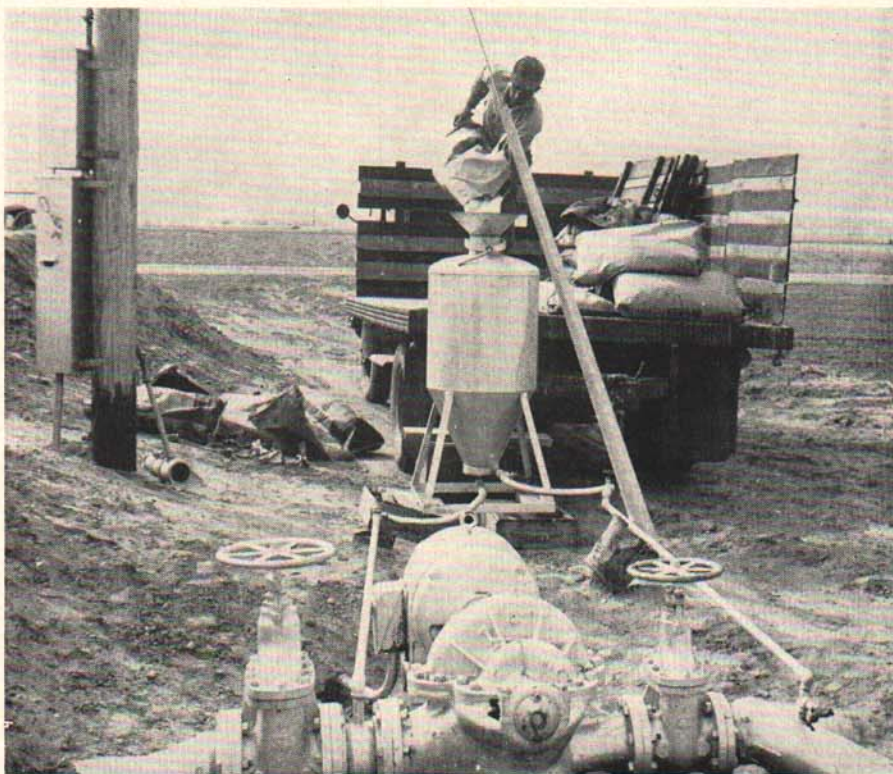
Fig. 6. One type of commercial fertilizer applicator which utilizes a pressure difference at a pump for feeding the solution into the sprinkler system.
