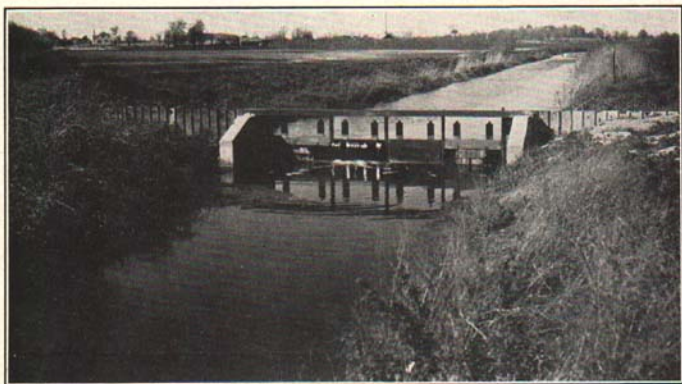
Fig. 1. Dam constructed to maintain water level in a large muck area. Note the use of interlocking sheet steel piling, which is driven deep to extend well out into the bank on each side. It is also driven across the ditch below the bottom of the gates. Concrete piers, concrete apron in the bottom of the ditch, angle iron braces welded into position, and four redwood gates complete the construction.
