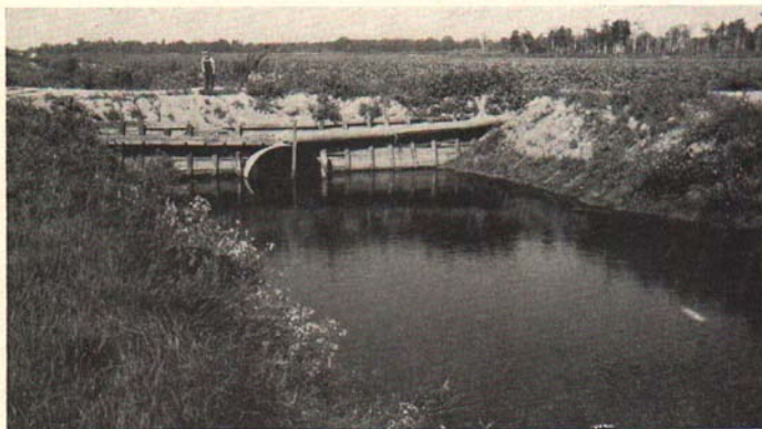
Fig. 4. View of secondary dam and bridge in the Chandlers Marsh drain, nine-tenths of a mile above the master dam shown in Fig. 3. This photograph was taken from the upper side, in late summer, before the retaining planks had been removed to lower the water level.
