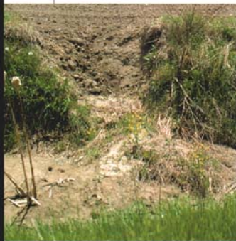
Ditch bank blow-out.
