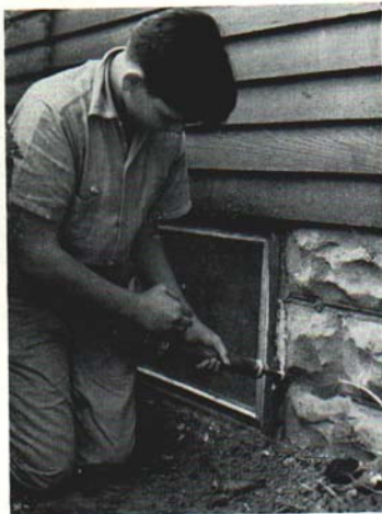
Fig. 3. Using a caulking gun to fill cracks between window frame and masonry wall with caulking compound.
