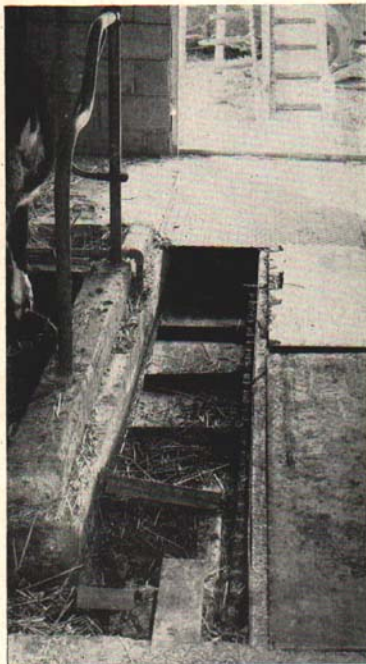
Fig. 17. Part of metal cover removed to show details of slats turning on themselves.
