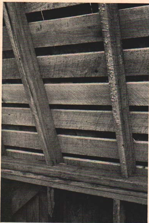
Fig. 13. An excellent roof deck, using sound uniformly sawed roof boards, properly spaced for nailing shingles. This construction is preferable to that shown in Fig. 14.
