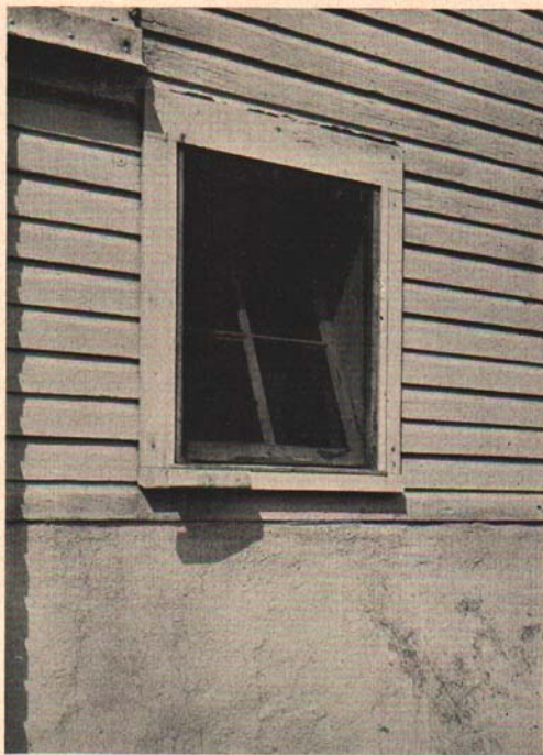
Fig. 8. Window construction without drip cap. This picture shows paint failure owing to moisture seepage around window frame and trim.
