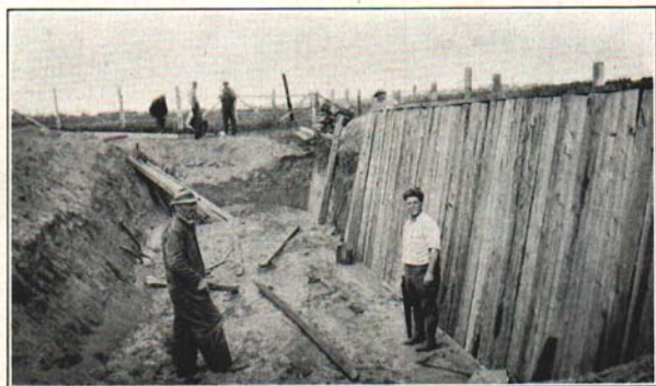
Fig. 5. A trench silo under construction in the Upper Peninsula. Cedar posts were used to line the inside.
