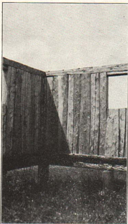
Fig. 12.—A barn basement being built of cedar logs set on end. The method of nailing them at the top and bottom between two long logs is clear. This type of basement was used in the barns shown in Figs. 17 and 18.
