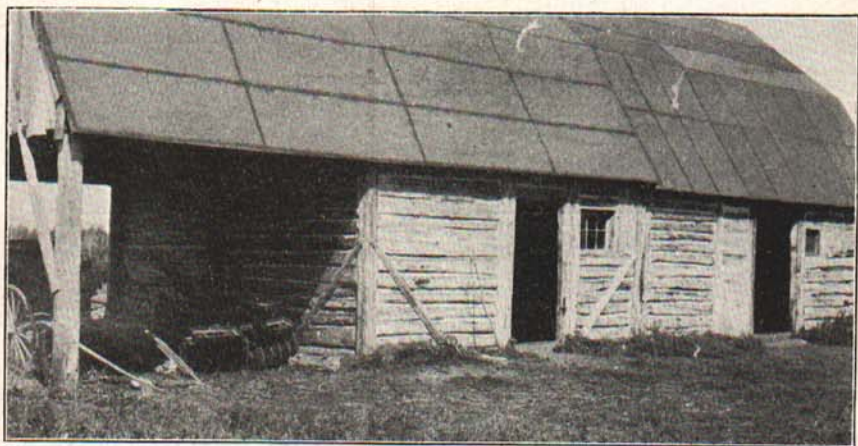
Fig. 19.—Barn made of cedar logs laid horizontally. It would have been better if more windows had been provided. The ends are toenailed to corner logs, instead of the method of notching and crossing used in other log buildings.
