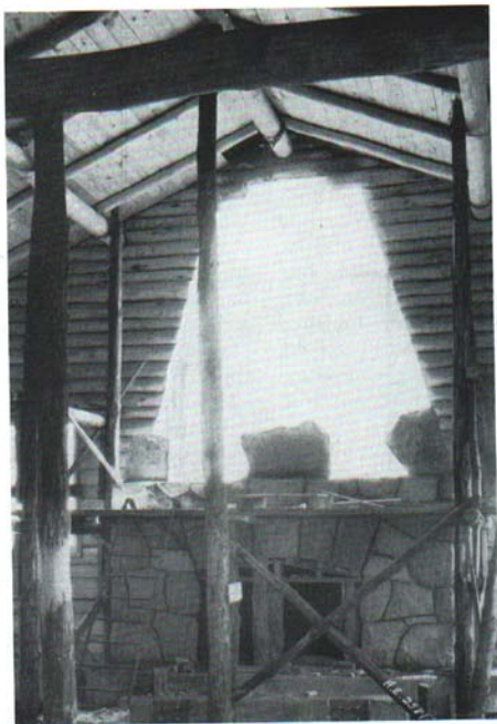
Fig. 19. Partially completed fireplace showing the placement of corner stones, framing for the fire-box arch and scaffolding.
