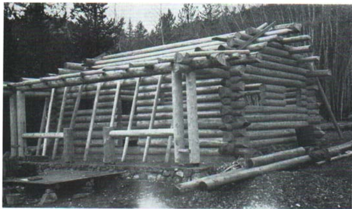
Fig. 13. Structural details of a horizontal log house. Rafters for the main roof lean against the wall.
