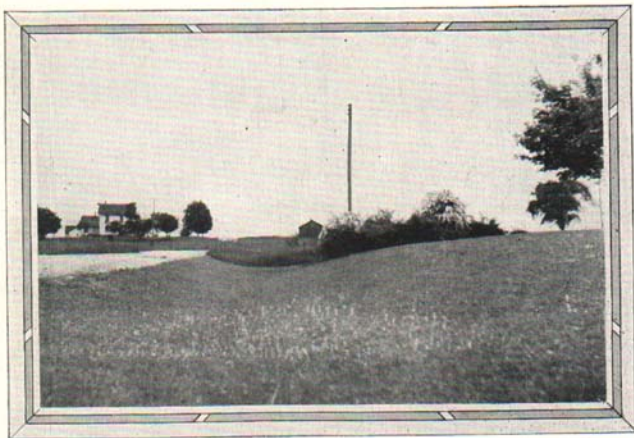
Fig. 18. After grading. Steep roadside banks should be cut back to form pleasing, flowing grades that will merge harmoniously into the surrounding landscape. (See Fig. 17.)
