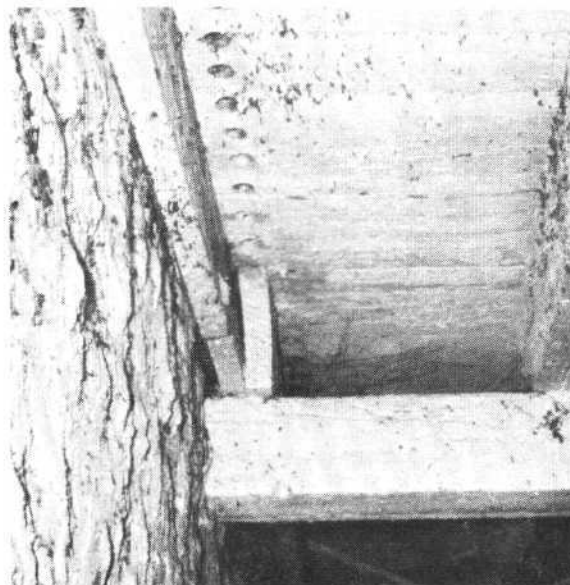
Figure 15. Three-inch diameter holes drilled in a ceiling to approximate a slot inlet.
