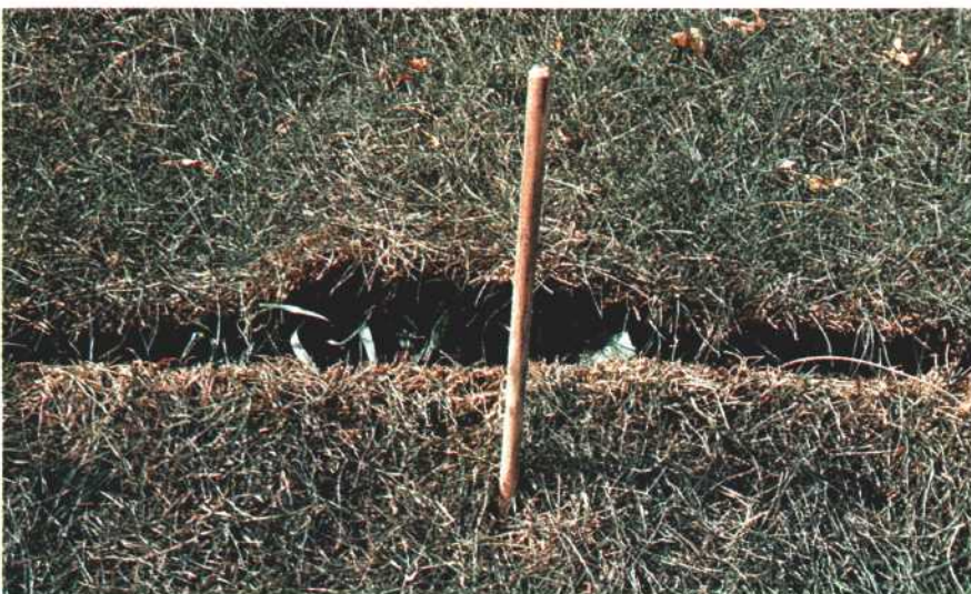
Sod can be staked to prevent slippage off of a slope., In this case the sod was stretched during installation and gaps were formed once the sod dried.
