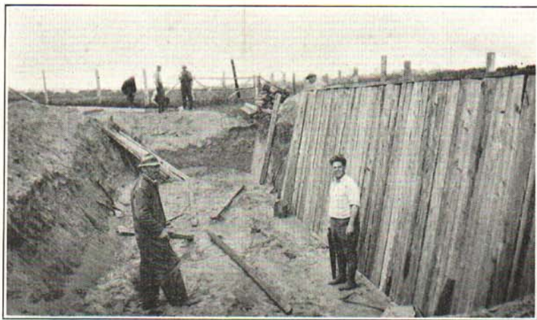
Fig. 4. A trench silo under construction in the Upper Peninsula. Cedar posts were used to line the inside.
