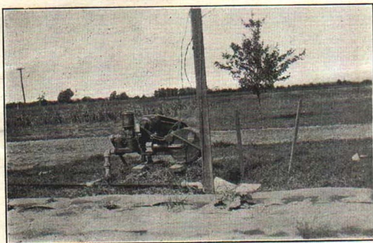
Fig. 15.—A piston pump operated with an electric motor pumping from 4 shallow wells.
