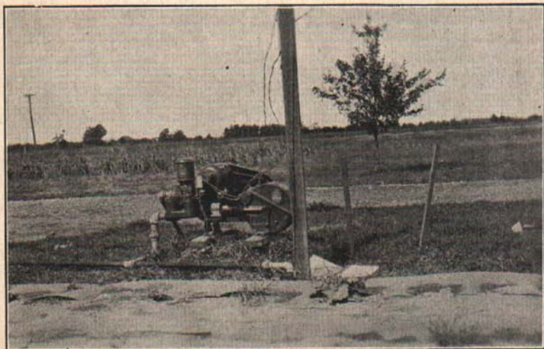
Fig. 15.—A piston pump operated with an electric motor pumping from 4 shallow wells.
