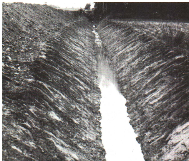
Figure 7. Open ditches can be dry part of the year or contain water. Engineers should design open ditch systems, but ideally, crop producers should maintain them. Seed grass to stabilize sides of ditch so that sedimentation does not reduce ditch depth.
