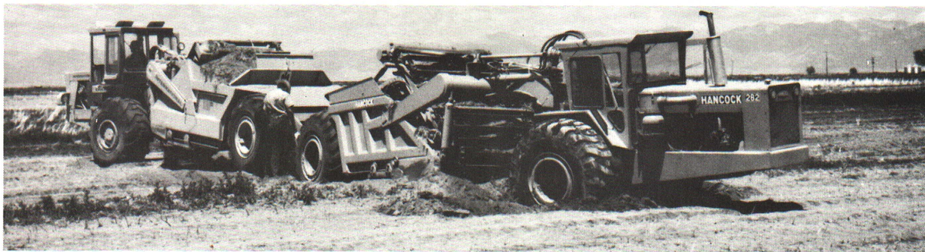
Figure 2. Land grading is a job for professionals. Here, an earthmover got stuck while preparing a field for surface drainage because the soil conditions were not correctly evaluated. Land grading should be used in Michigan with caution because surface soil layers are usually thin. Soil physical and chemical problems are common when subsoil is exposed.
