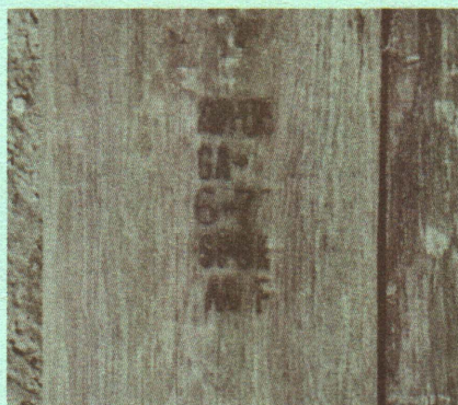
Fig. 2. Brand on piling treated with CCA preservative.
