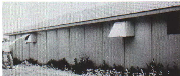
Figure 2. The hoods and fans on this hog barn were completely rusted and corroded through in about 3 years. Periodic maintenance is required to minimize this kind of deterioration.
