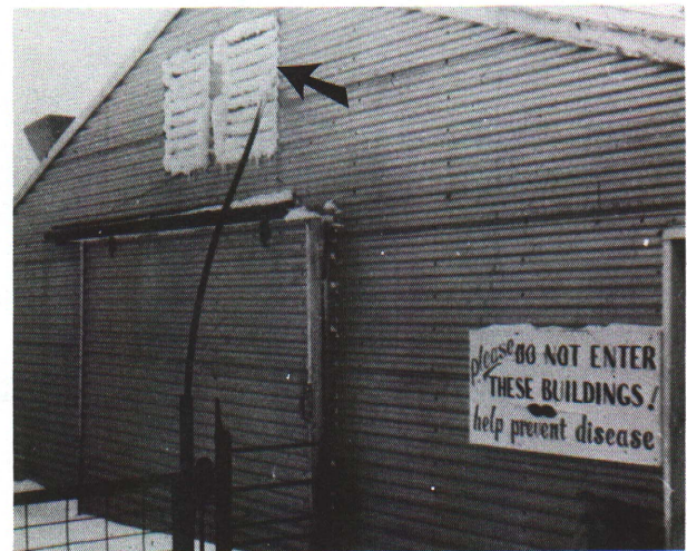
Figure 10. The variable-speed exhaust fan operated at too slow a speed in this farrowing barn. High winds sucked moist air from inside the barn back up through the ceiling inlet into the attic space. There it condensed into frost.
