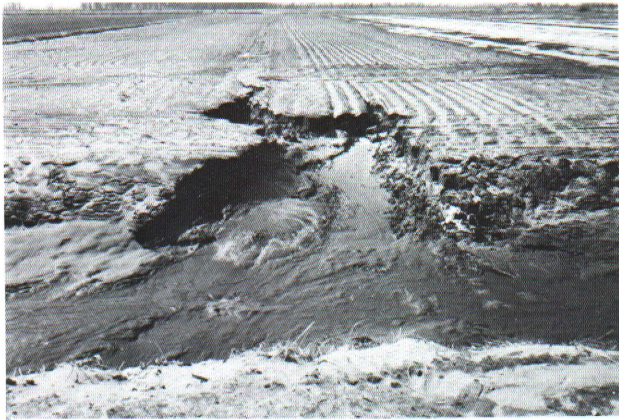
Figure 3. Shallow gully erosion on flat land in Saginaw County. Erosion is occurring where water enters road ditch. This resulted after road was improved. No vegetation was ever established on the ditch banks.
