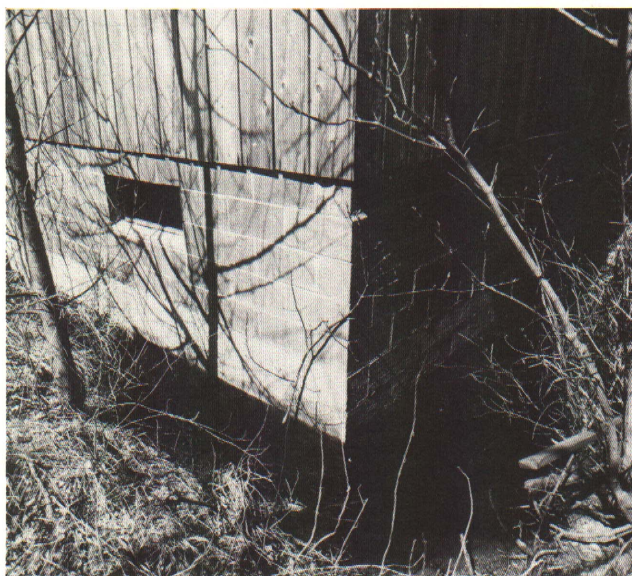
One of many soil problems to be aware of—high water table resulting in water around foundation and in basement.
