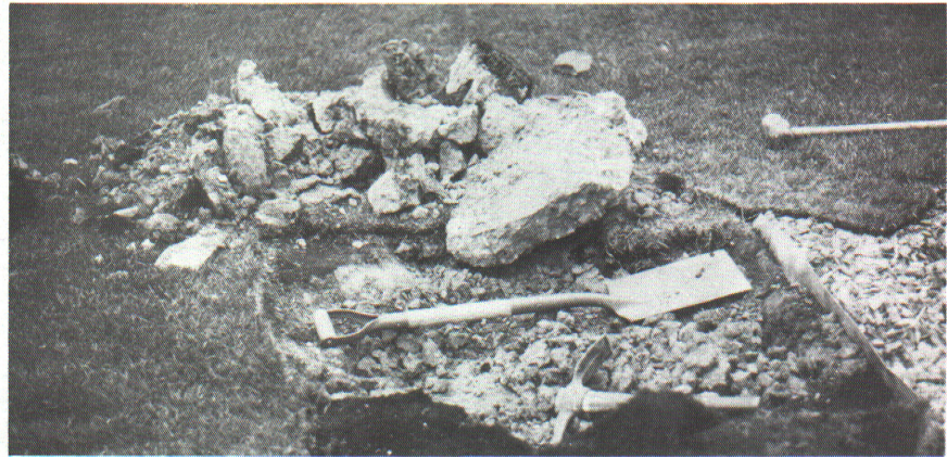
Problems arise when buried debris is not removed prior to establishment.
